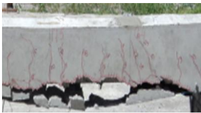
Fig. 1 - Detachment of protective milking concrete in the area of anchor lamella
