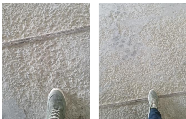
Fig. 1 and 2 Defective zones of cell 4
