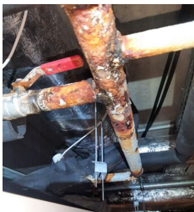
Fig. 1. Corrosion-damaged section of cold-water piping in a building
