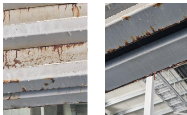
Fig. 5 and 6 Corrosion in steel entrance doors
