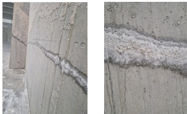
Fig. 3 and 4 Defective wall concrete
